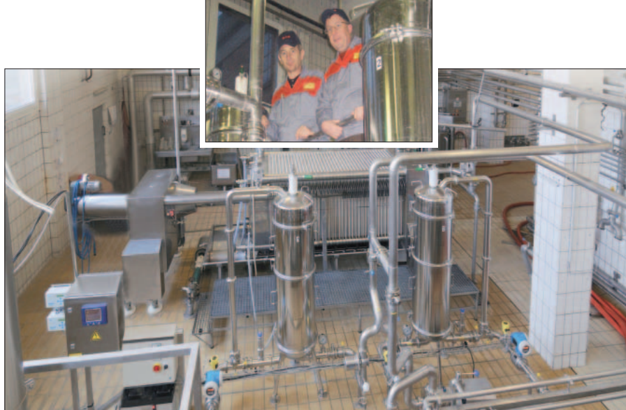
Fig. 6: Filter cellar with kieselguhr filter in the background; new installed SUPRApak housings in the foreground. Small photo: Technical Manager Jean-Marie Kessler (right) and Brewmaster Ernewein Roger
