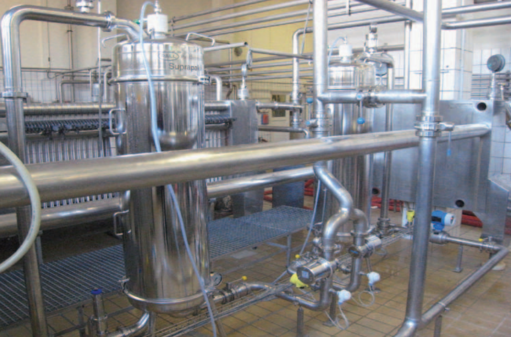
Fig. 5: SUPRAPak installation between the beams of the dismantled sheet filter as an interim solution during qualification time, clearly to be seen the essentially smaller place requirement.
