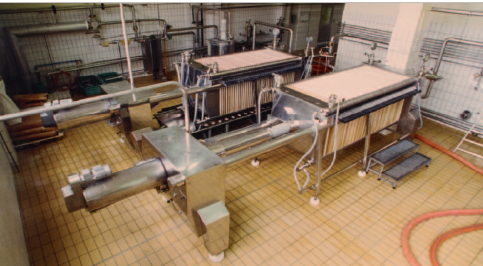
Fig. 3: Filter cellar prior to the SUPRApak tests, kieselguhr filter (background), sheet filter (foreground).
